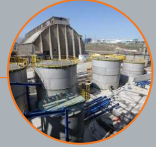
Stok Tank Storage Tank
