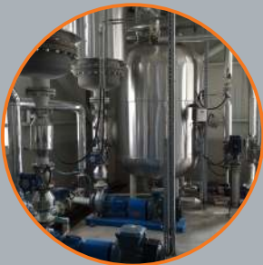
Proses Tank Process Tank
